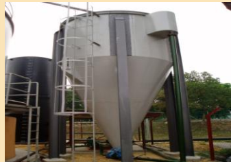
SETTLING TANK Sludge separation
