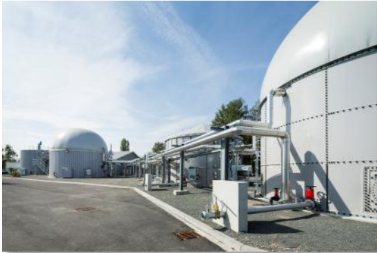
Biogas pilot plant
