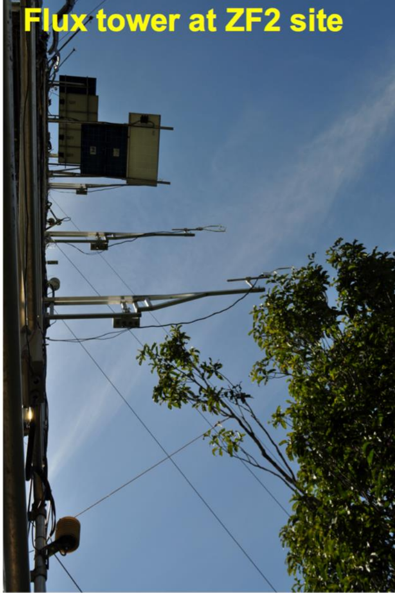
Sonic anemometers on the tower
